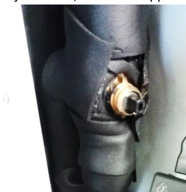
1 – Links van de boiler
